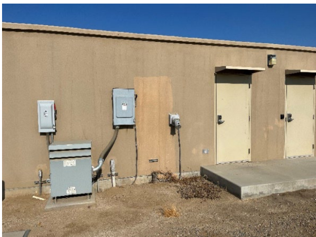
Figure 2. Exterior Headend Doors
