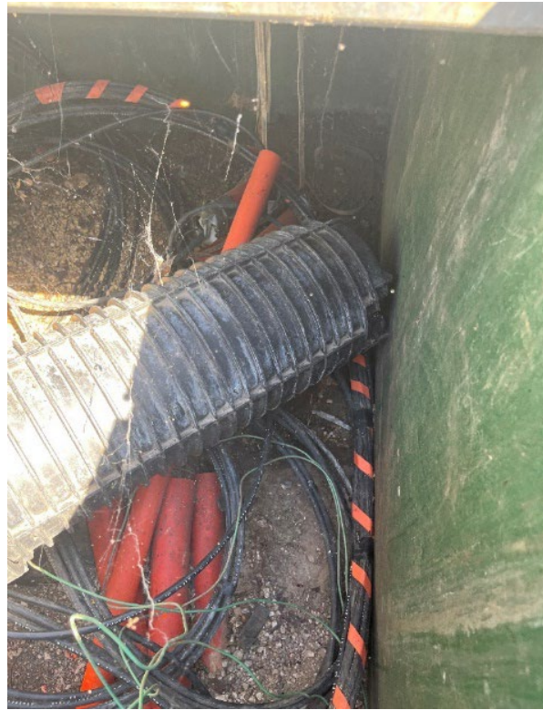
Figure 20. Splice Case in Vault
