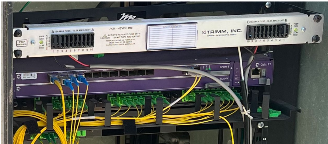
Figure 16. Gossamer PON Equipment
