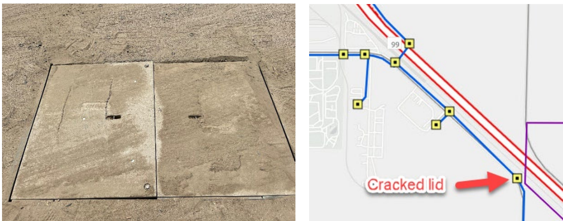
Figure 18. Cracked Vault Lid
